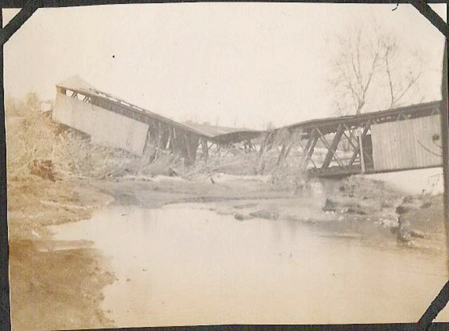
Bridge after 1913 Flood
